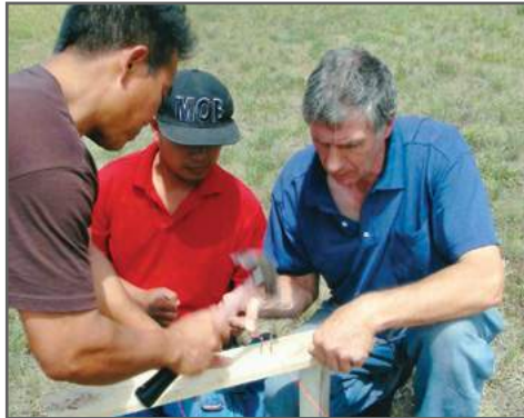
Retired pastor John Billingham worked with teams of volunteers to complete the building
